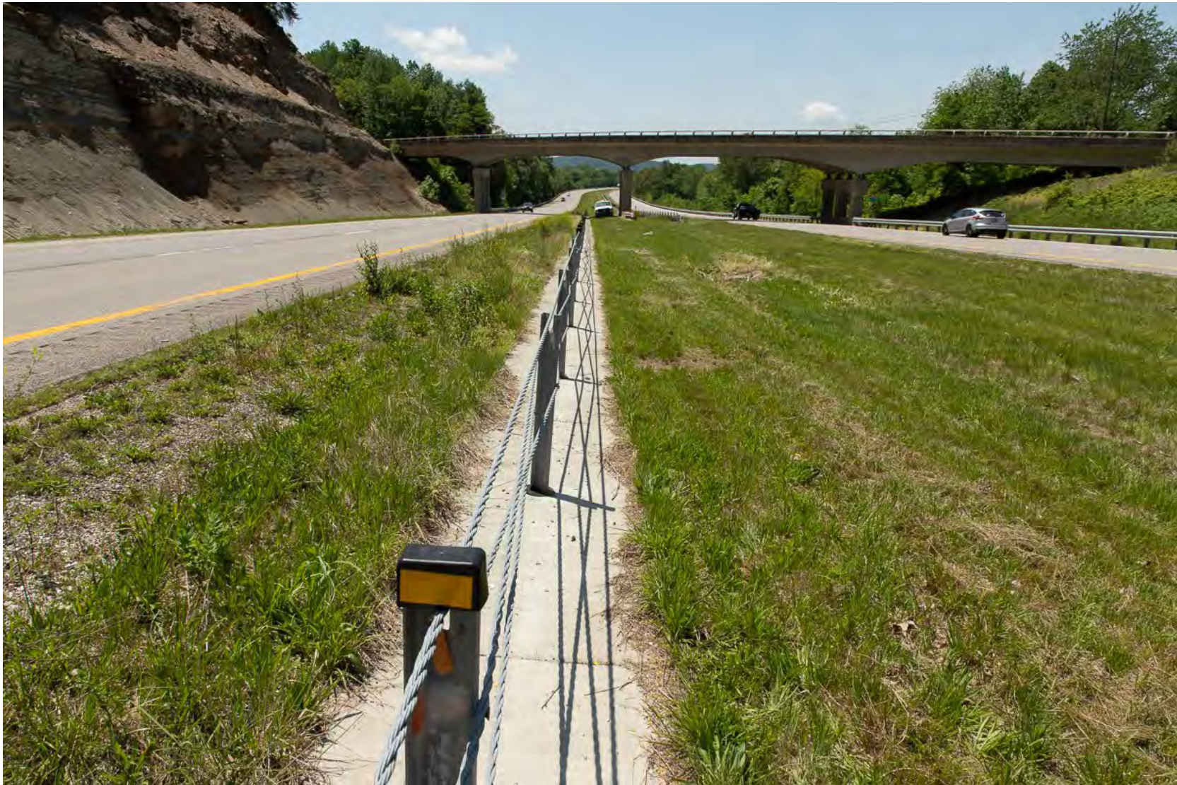
Figure 5: View of Plots in the Cable Barrier Trial on May 19, 2022 (357 Days After Treatment)
